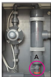
Reactor Leakage Device
